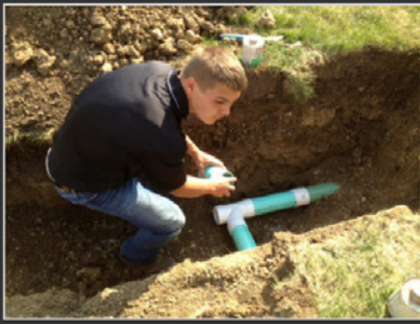
Taylor Layne, of Manteno, installs the pipes that will send clean water from the new wastewater system into a storm drain behind the industrial condominium building in New Lenox. | Susan DeMar Lafferty/Sun-Times Media
