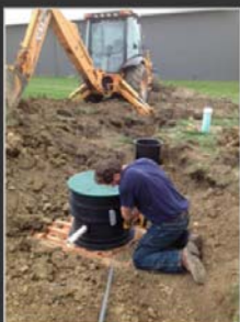
Ray Tebo, of New Excavating Technologies, installs Will County's first BioBarrier membrane bioreactor wastewater system in the Old Plank Industrial park in New Lenox. | Susan DeMar Lafferty/Sun-Times Media
