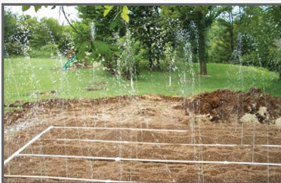
The bottomless sand-filter system installed by attendees of the KSFA "Classroom Training" workshop.
