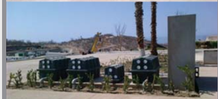
Control Panel house and Blowers for the MyFAST® system.
