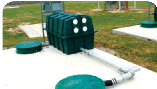
Bio-Microbics FAST System installed in the Dawn Community in Caroline County, VA.
